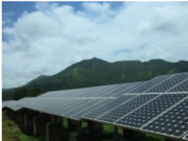
Tata Solar Power makes modules and develops projects. Source: Tata Solar Power.
